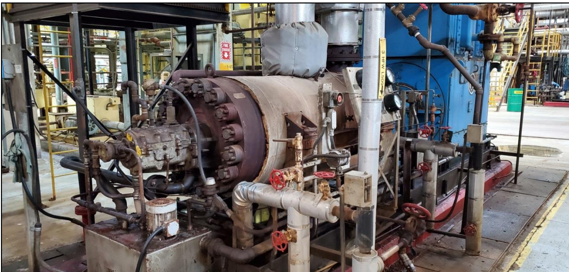
Figure 1: Unit 3 Boiler Feed Pump West
