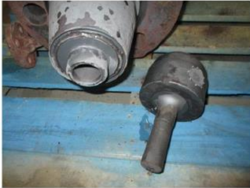
Figure 3: Control Valve with Broken Stem
