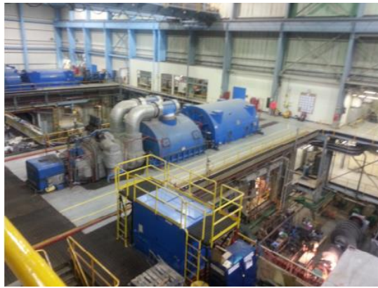
Figure 1: Holyrood TGS Unit 2 Turbine Generator
